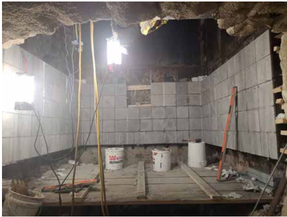
Completed installation of the first section of the cooler throat and kiln hood walls with the HASLE precast modular lining system.
