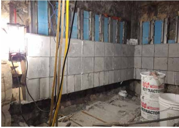
Installation of HASLE precast modular lining in the cooler throat and kiln hood at the Paulding cement plant.
