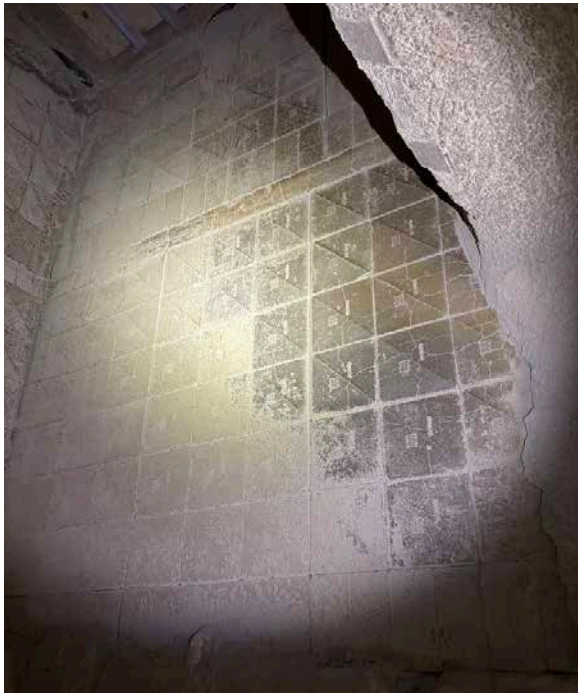
Inspection during a scheduled shutdown in March 2025. The precast lining remains in service and continues to perform as intended. In 2026, the lining remain in service.
