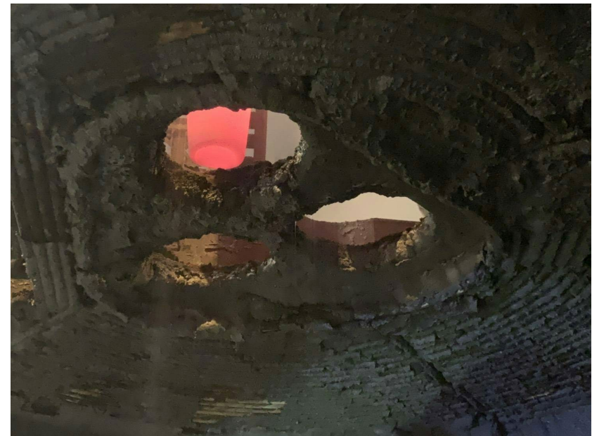
After 420 cycle heats or around 600 hours with 1550-1570°C operating temperature
