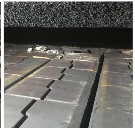
Elements installed in walking beam furnace
