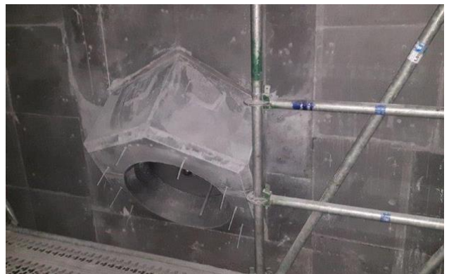
HASLE D39A and D39A-EF casting around nozzle
