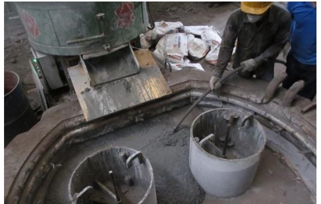
Installation HASLE D1700A
