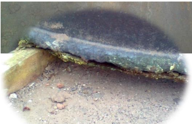
Bottom of previously installed Steel Vortex Finder after 8 months
