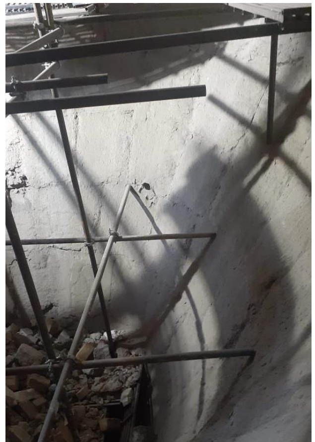
D52A in Dust Settling Chamber at inspection after 4 years
