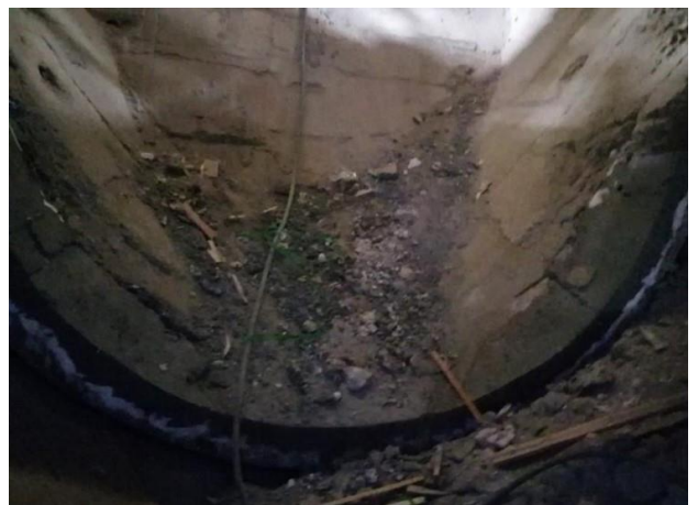
HASLE D59A-ht in Inlet Cone after 12 months. Final lifetime 24 months.
