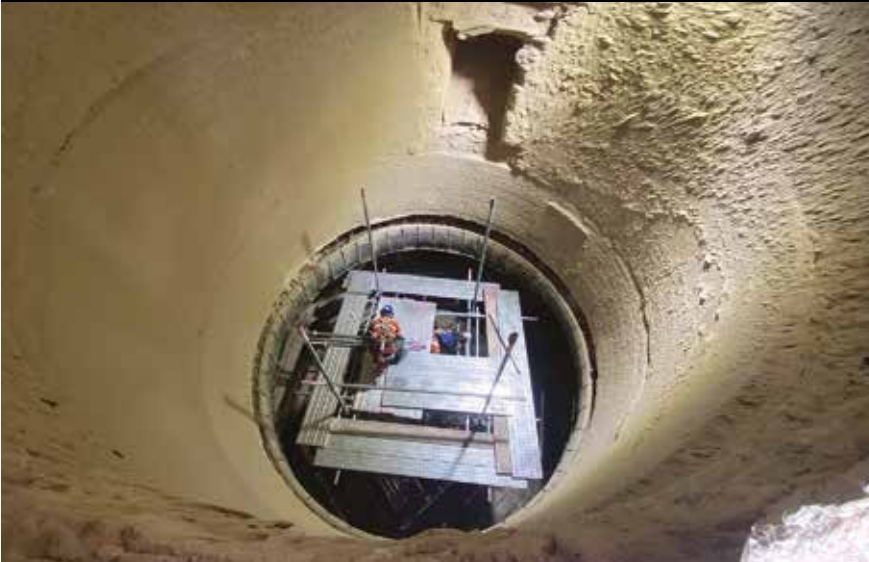
Figure 2: as the vertical bull nose area is located high above the manhole in the cyclone at the Thai cement plant, scaffolding is needed to reach the area
