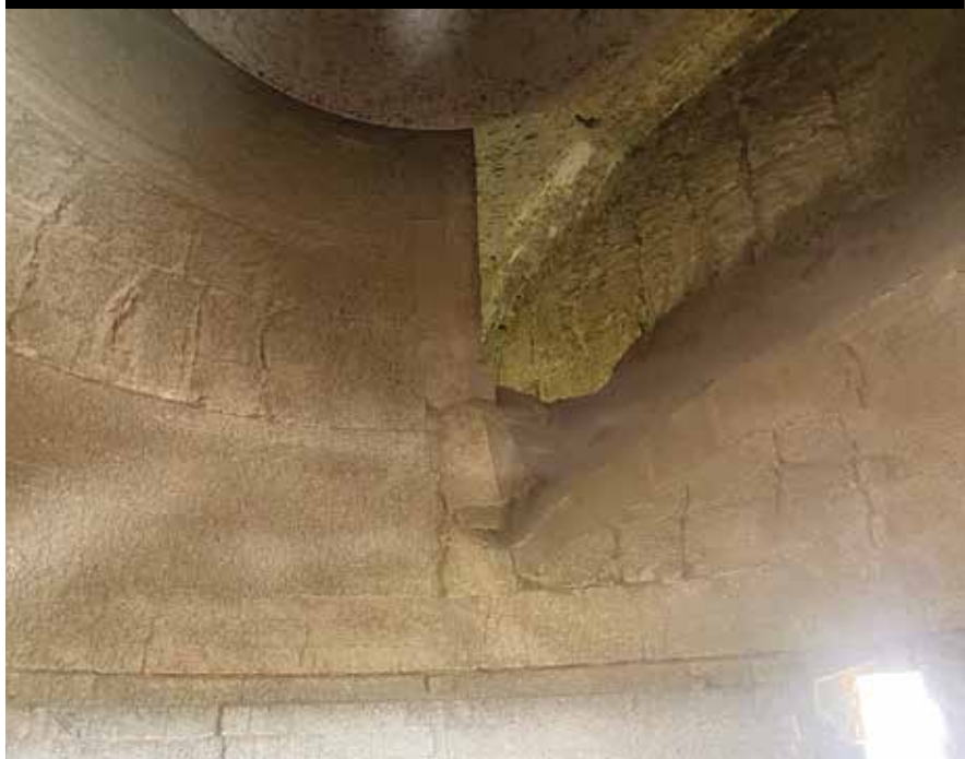
Figure 4: HASLE modular lining in the middle stage cyclone five years after installation at the Thai cement plant
