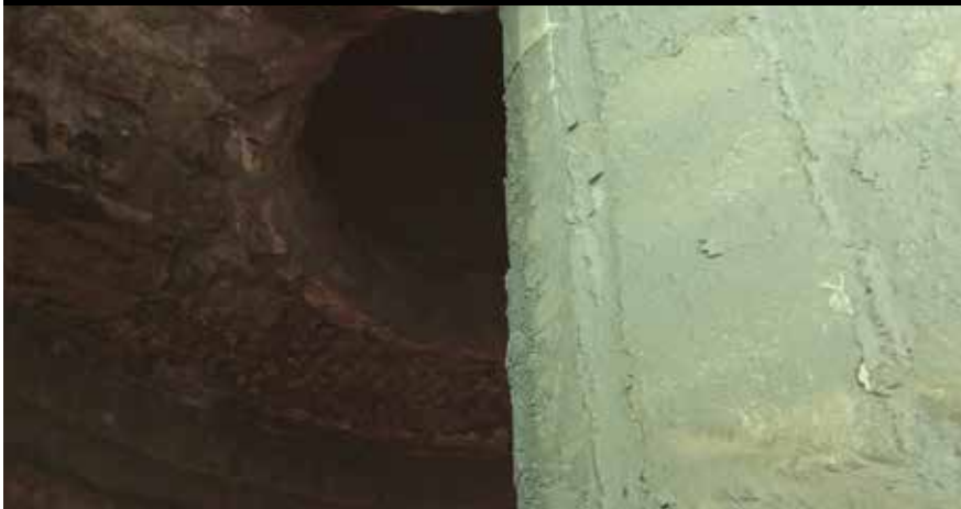
Figure 3: HASLE modular lining in the lowest stage cyclone 2.5 years after installation at the Thai cement plant
