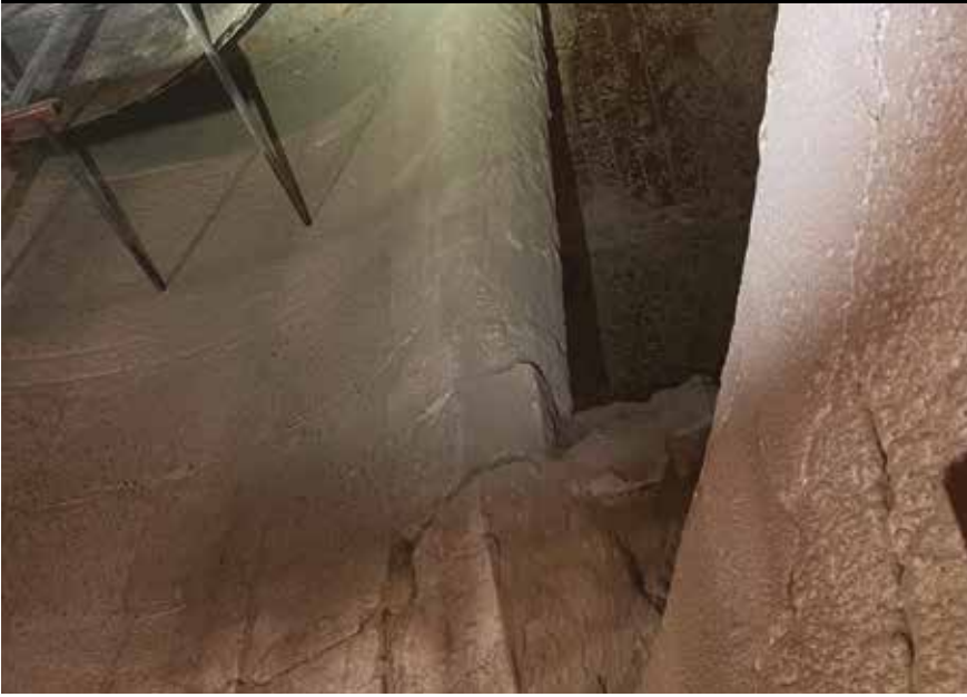
Figure 5: HASLE Modular Lining in the middle stage cyclone in 2022, more than six years after installation at the Thai cement plant. It is still in good operating condition
