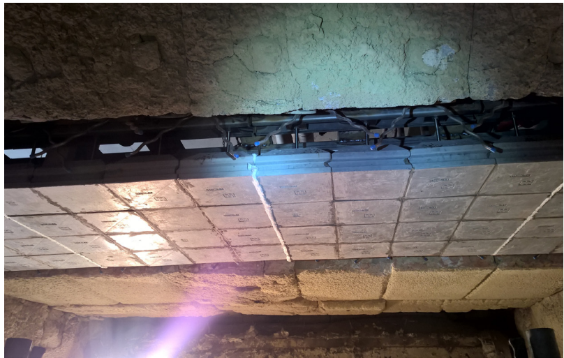
HASLE Modular Lining during installation in 2018 in the hot zone of the cooler roof at a German cement plant. Thermal expansion joints are incorporated at every metre.
