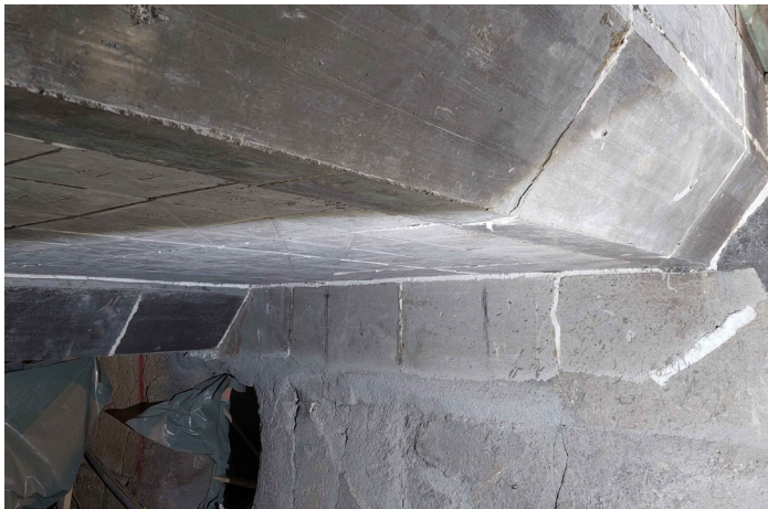
HASLE Modular Lining installation at Holcim Zementwerk Retznei, Austria. The adaptable anchoring system allows for a lining thickness as low as 185 mm. Looking to increase the cross-sectional area of the clinker cooler, it resulted in a gain of 420 mm in roof height compared to its previous solution.
