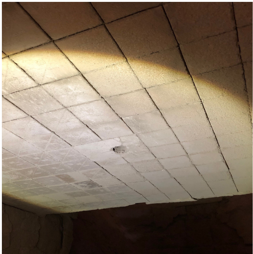
The same HASLE Modular Lining in the hot zone of the cooler roof in October 2023, five years after installation.
