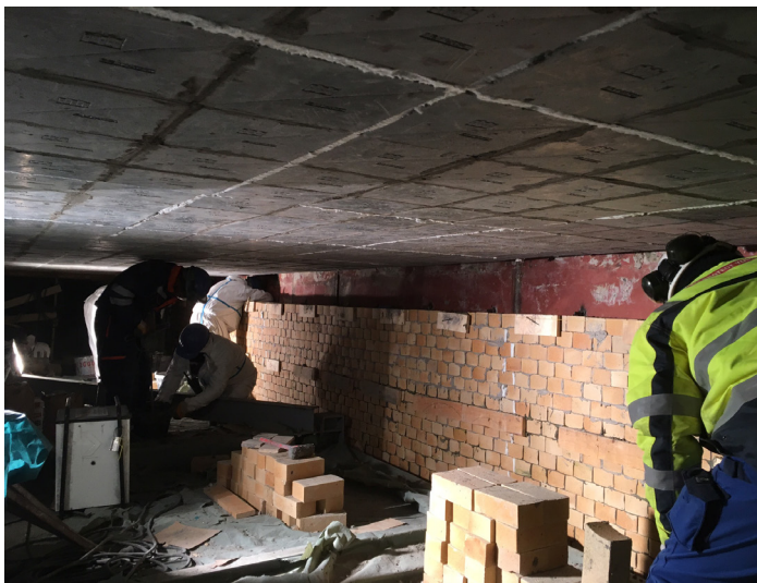
40 m 2 HASLE Modular Lining being installed in the cooler roof at German cement plant in 2018.
