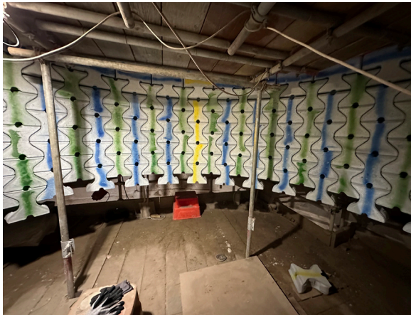
Assembling the GEN3-CVF; the top row of ceramic elements is placed on the brackets of the steel support ring; the remaining elements are suspended from the elements in the top row.
