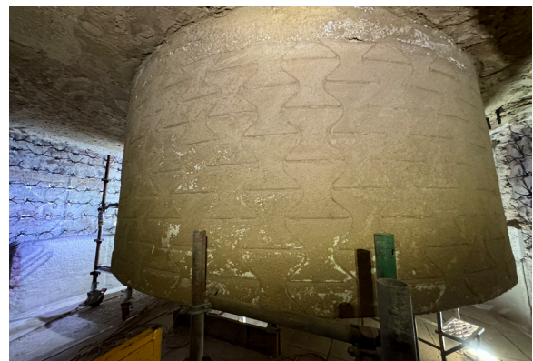
After a year of operation, the CVF in the lowest stage cyclone at the ADBRI Birkenhead plant underwent a comprehensive inspection. It was found to be in excellent condition with no visible damage, leading to the decision to continue its operation.
