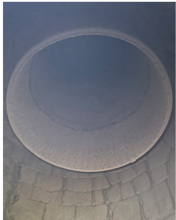
The CVF at the ADBRI Birkenhead plant after four months of operation.
