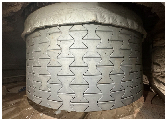
The CVF (Gen3) fully assembled in the lowest stage cyclone at ADBRI's Birkenhead plant.
