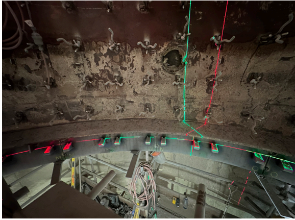
The alignment and level of the steel supporting are verified, prior to the installation of Ceramic Vortex Finder in the lowest stage cyclone at the ADBRI Birkenhead plant in Southern Australia.
