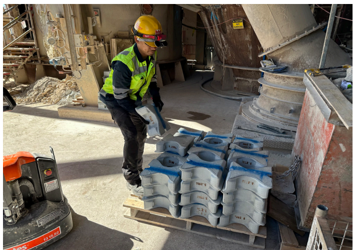
Due to the individual elements' low weight of 6 – 19 kg, no heavy lifting equipment is required for handling, and it is possible to use the existing manholes for the installation.
