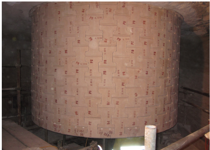
Developed in the 1980s by HASLE Refractories, the first generation of the Ceramic Vortex Finder was also installed at the ADBRI Birkenhead plant. Here an installation in 2009 is shown.
