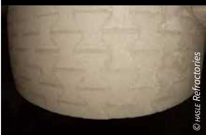
The CVF in the lowest-stage cyclone after one year of operation at the German cement plant
