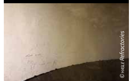
The CVF in the second-lowest stage cyclone after three years of operation at the German cement plant
